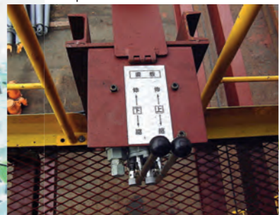
操作盤 Operation Board
